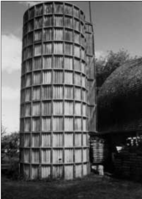
Asbestos silo in Jefferson County. Asbestos was used as silo construction material during World War II.
